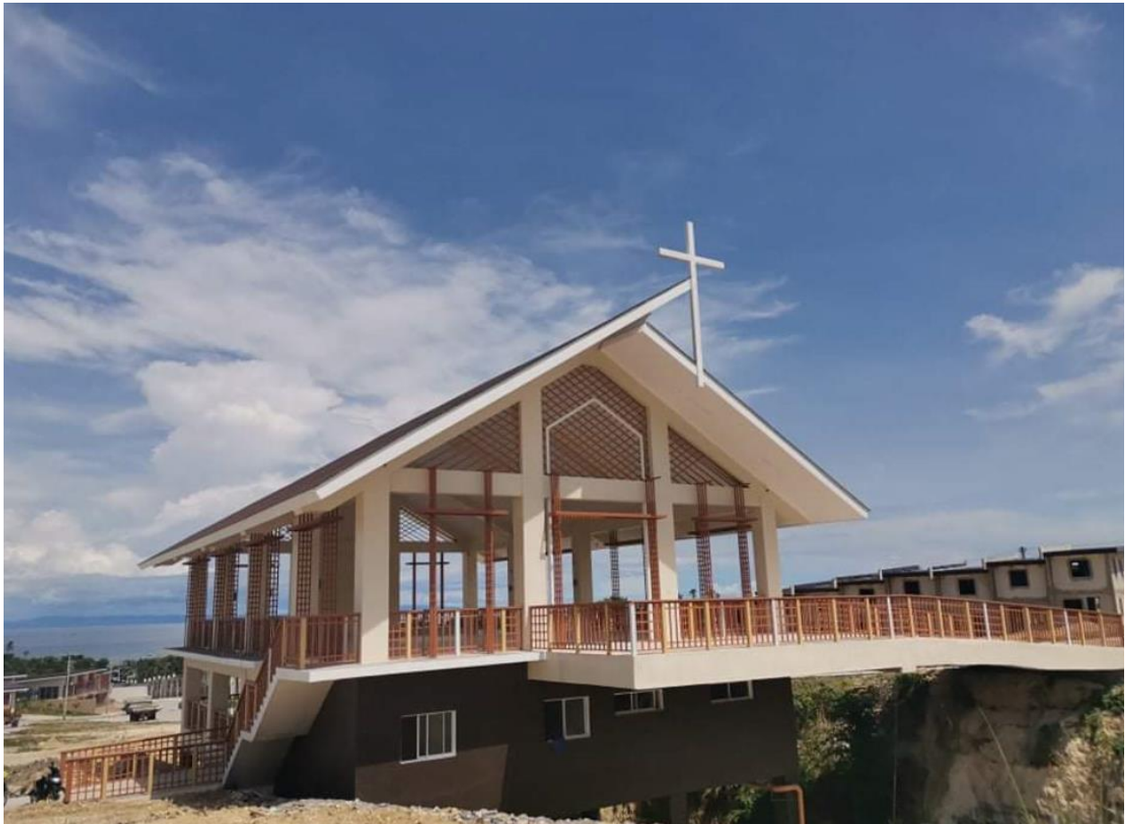
Latest construction updates of the Casa Mira South club house with its own chapel.
